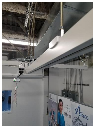
Figure 2: Shows the installed Amico track in a gantry system.
