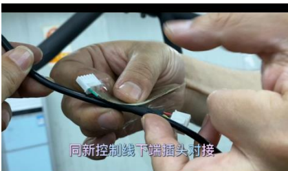
1. Unplug the old communication wire from the console and fix with the new communication wire by tape
